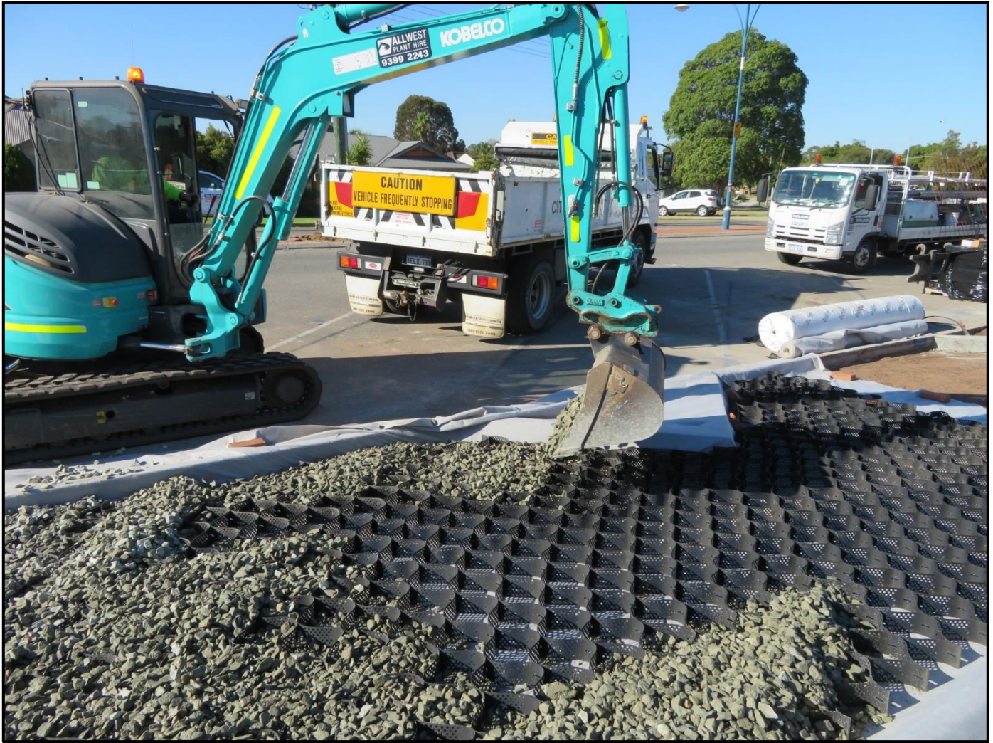
Figure 14. Example of GeoWeb product being installed within Epsom Avenue , Belmont – Image source City of Belmont (WA)
